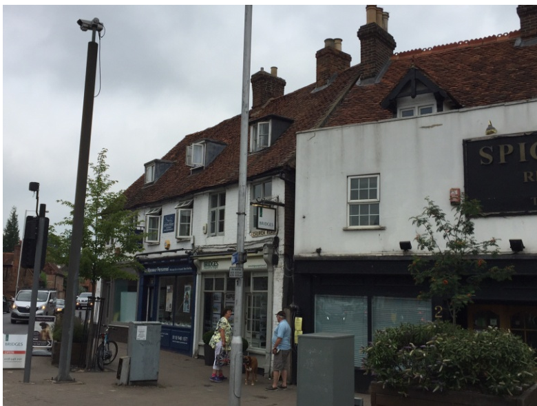
UPVC window replacements in a listed building. Opportunities should be sought to reverse such damage when maintenance, replacement or alterations are carried out. In the foreground a utilitarian mast, pole and cabinets also detract.
