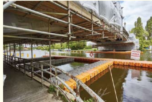
Scaffolding allowed for a detailed inspection which identified hollow points across the whole structure. (Photo: VolkerLaser)
