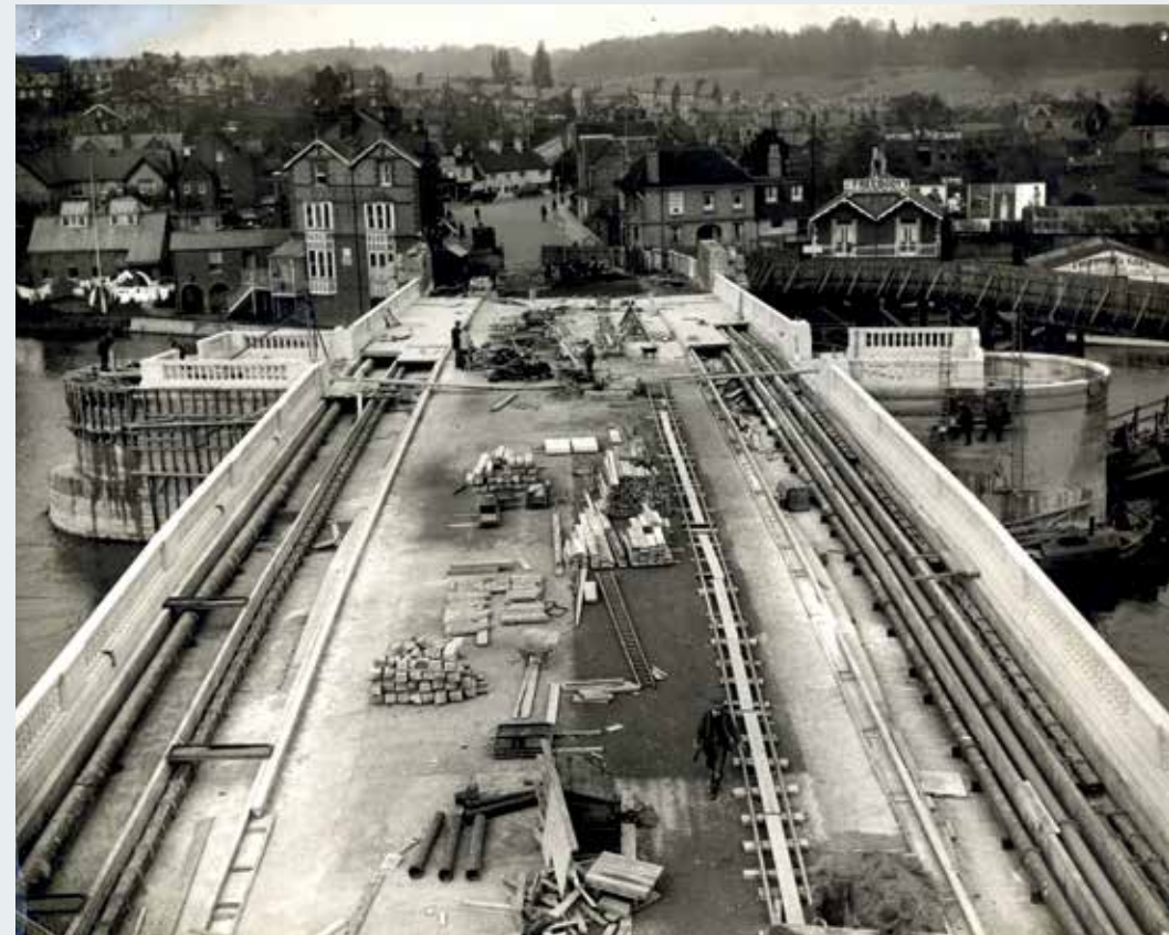
▼ Utility services are laid under the footpaths. The Crown Inn was remodelled to accommodate the bridge. Next to it on the main bank are Freebody's boat premises. Image: Reading Library Services
