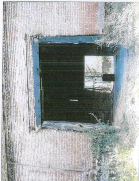
Plate 4 - North elevation doorway. Evidence of an overdoor roof is shown across the lintel.
